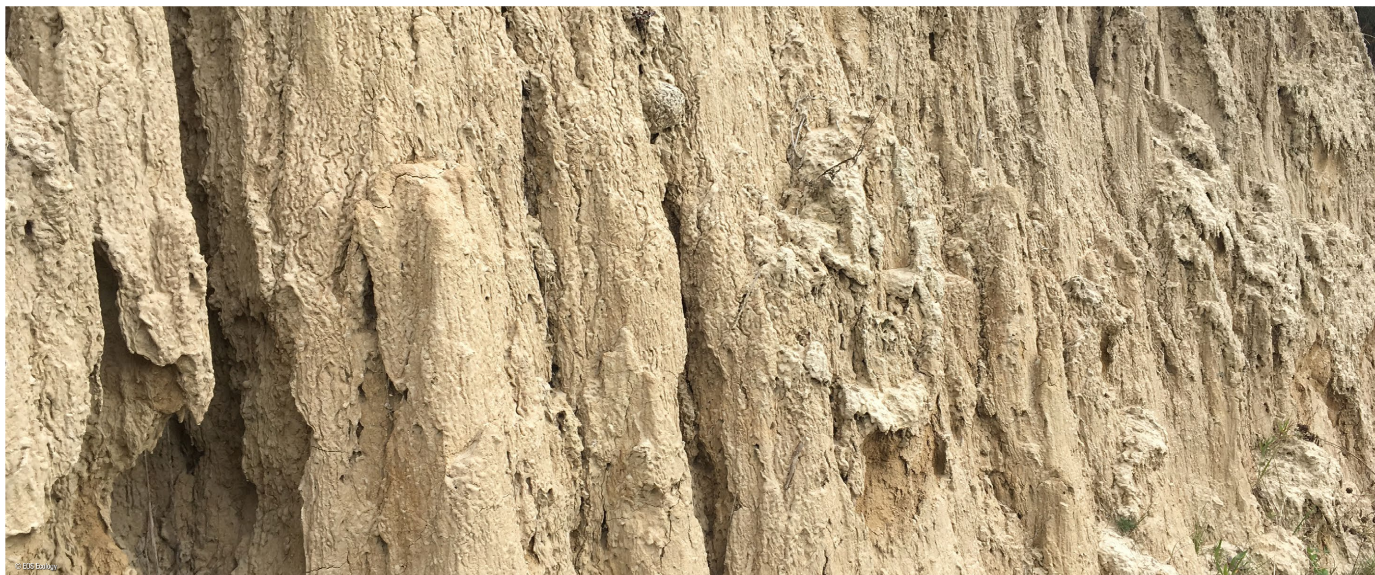
Loess subsoil eroding on a cut face in the Port Hills (soil order: Pallic (P), soil group Fragic (PX)).
